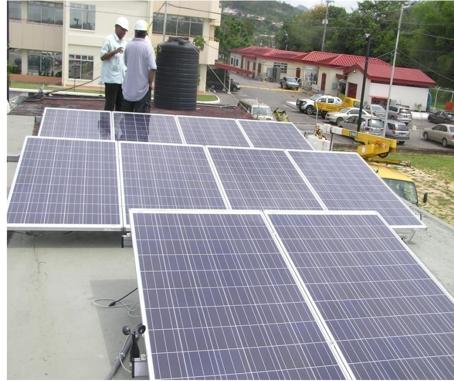
Trinidad and Tobago Electricity Commission Mt. Hope Compound (2 kW)
